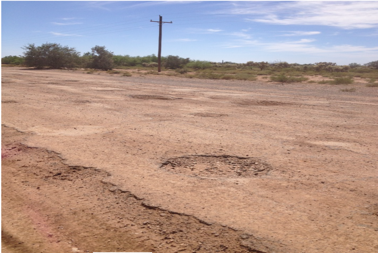
Figure 3: Potholes in [REDACTED] access road Source: OIG photo
