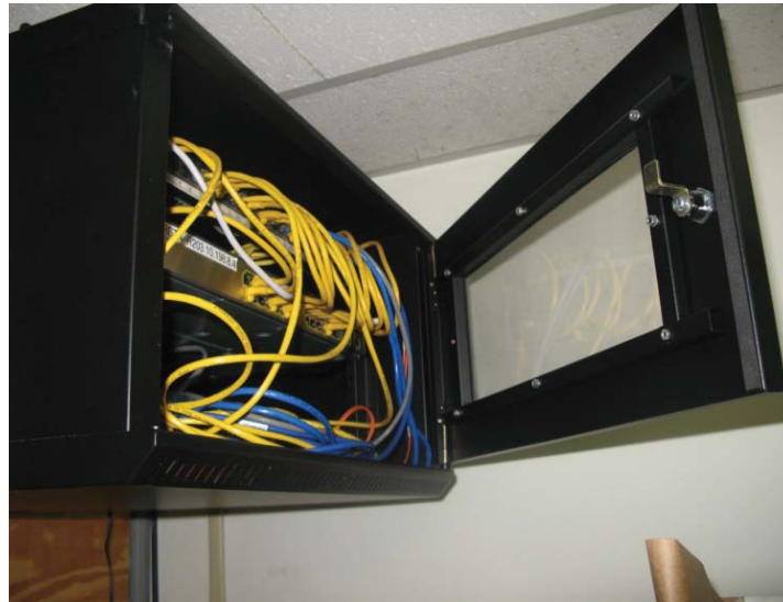
Figure 4: Exposed and Unsecured Network Equipment
