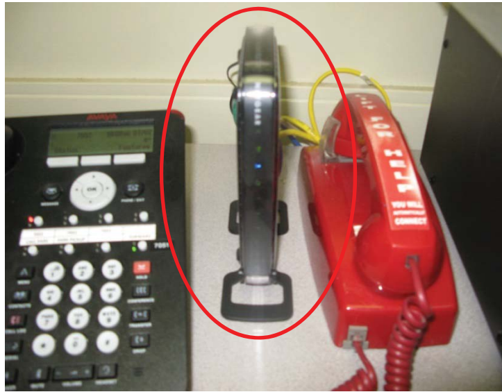
Figure 6: Exposed and Unsecured USCG Wireless Router
