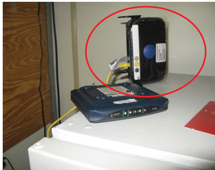
Figure 5: Exposed and Unsecured USCG Wireless Router
