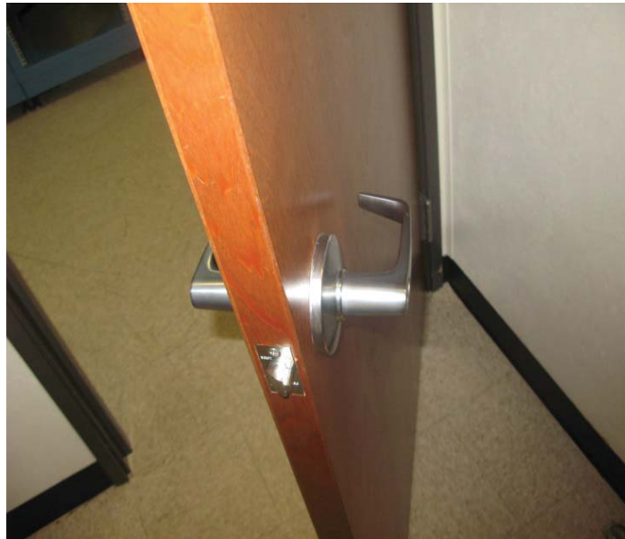
Figure 2: Network Equipment Room Door with No Access Card Reader
