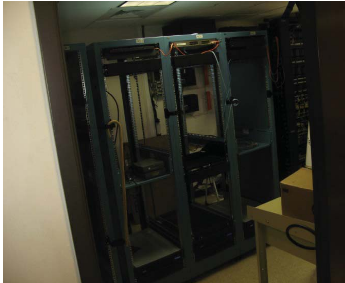
Figure 1: Unlocked USCG Network Equipment Room
