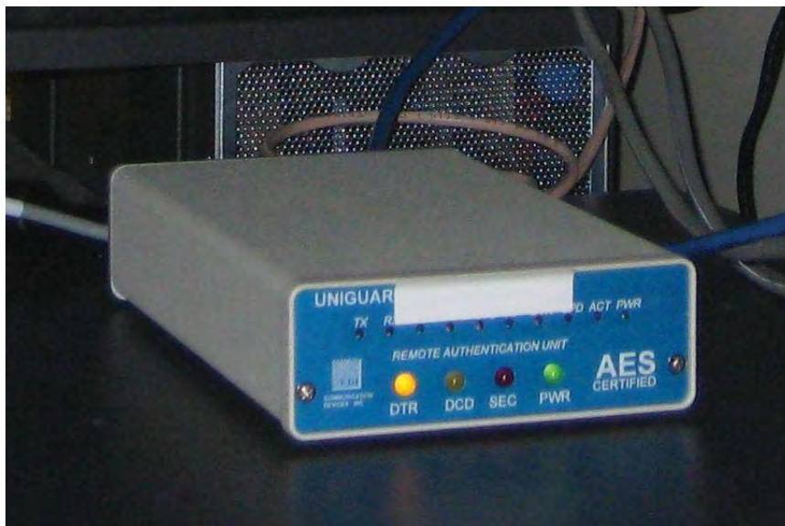
Figure 1. Out-of-Band Modem Device Attached to a DHS OneNet Router
