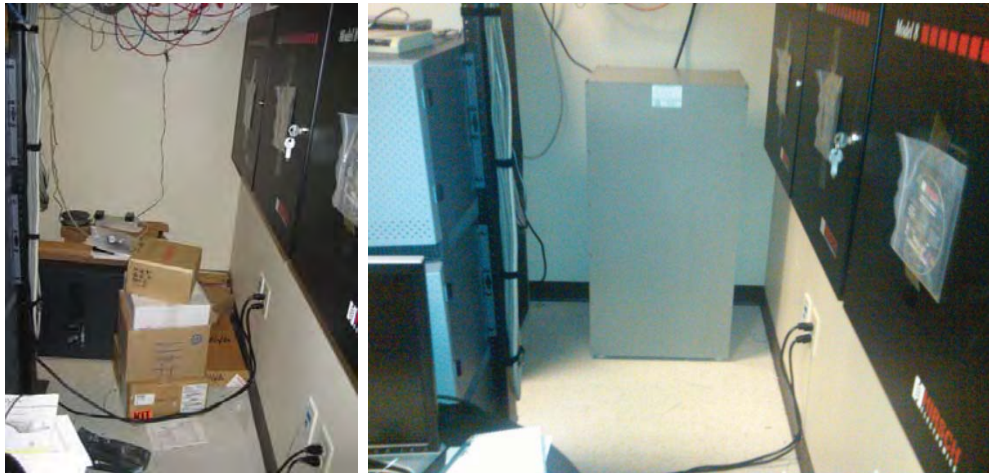
Figures 3a and 3b. Before and After Pictures of Storage in Room With ICE IT Equipment
