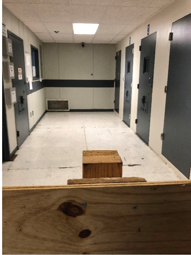
Figure 1. The Cordoned-Off Section of the Segregation Building Separated by a Plywood Barrier, Observed on April 26, 2022
