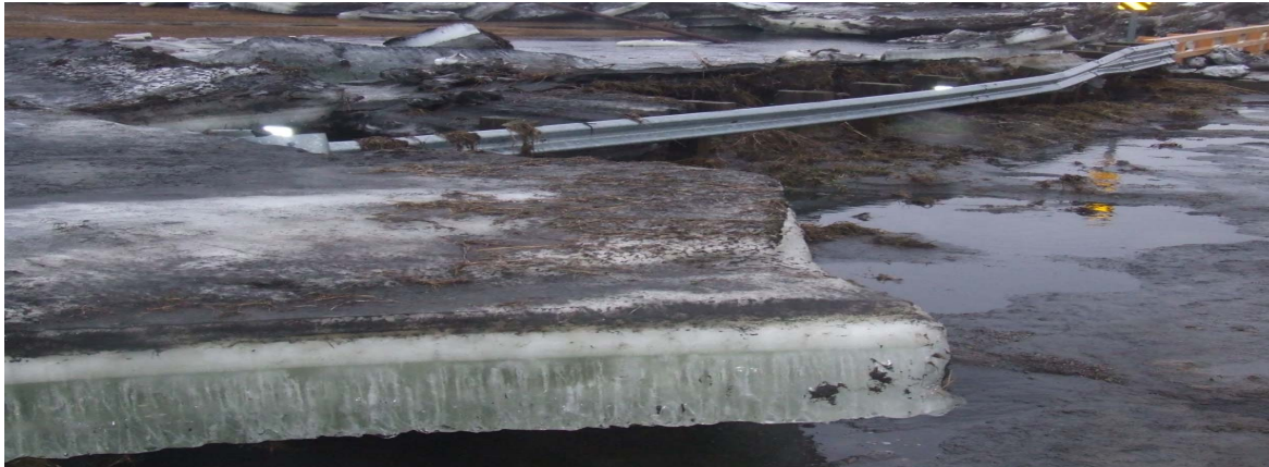
Figure 1. Ice Damage on North Dakota Road Source: North Dakota Department of Emergency Services
