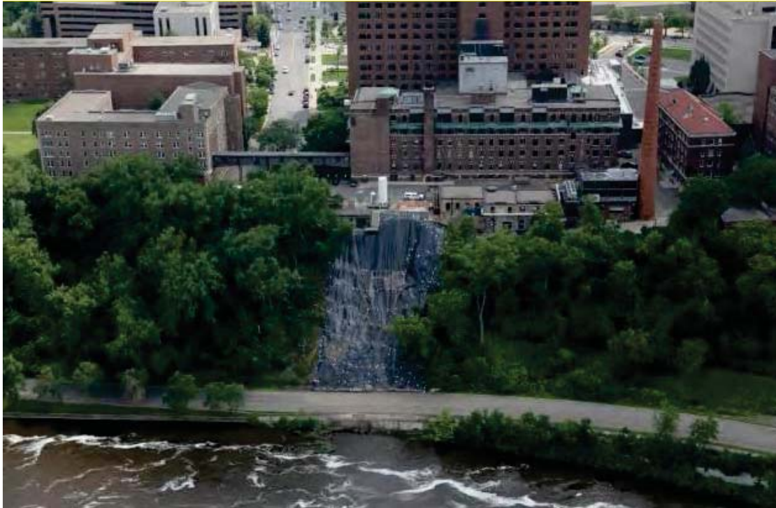
Figure 1: Minneapolis Slope Failure
